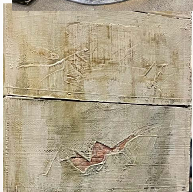
Above: Building walls have layers of texture, with plaster peeling in areas to reveal brickwork underneath.
